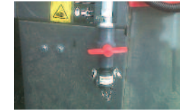
Filling and drain point
